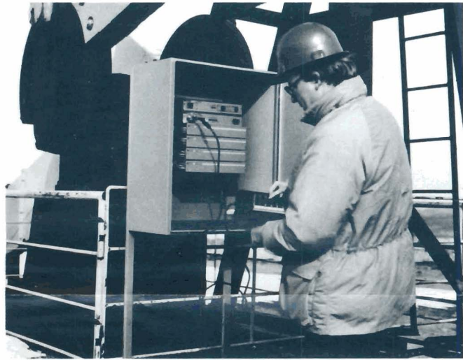
For oil pump surveillance and control, the HP 48000 RTU Measurement and Control Unit program can be modified easily in the field.
